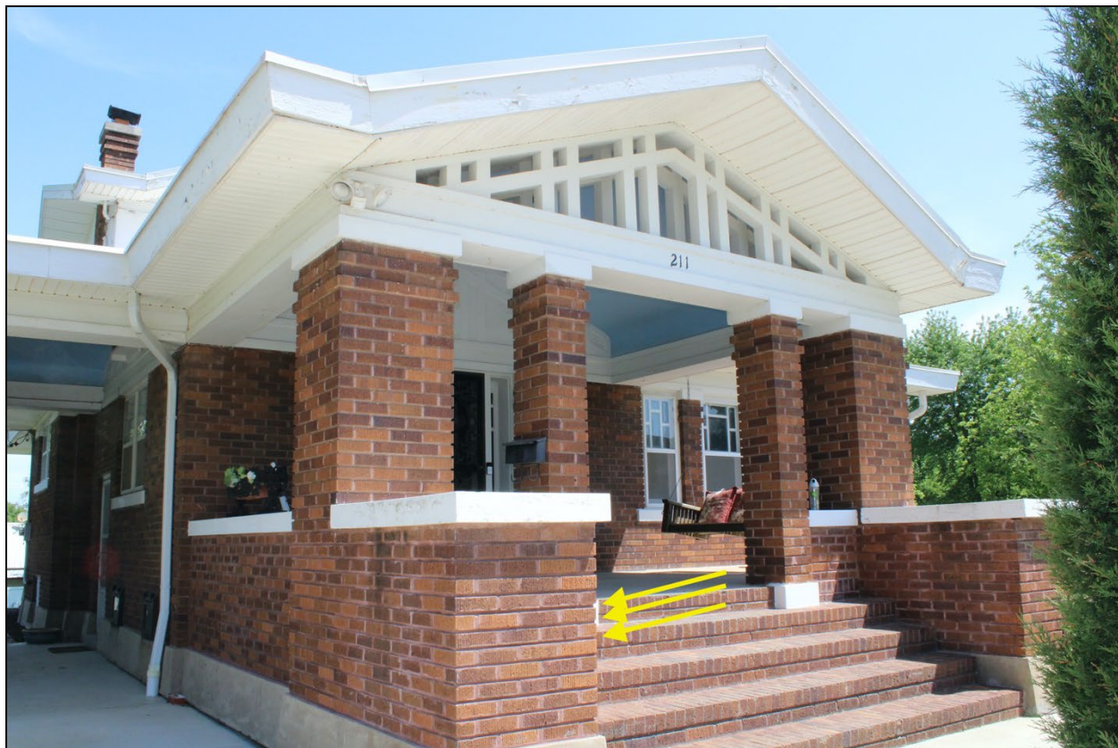
Figure 18: Main facade, detail of horizontal emphasis of masonry joints, pointed out by yellow arrows; view facing northeast, 2022.
