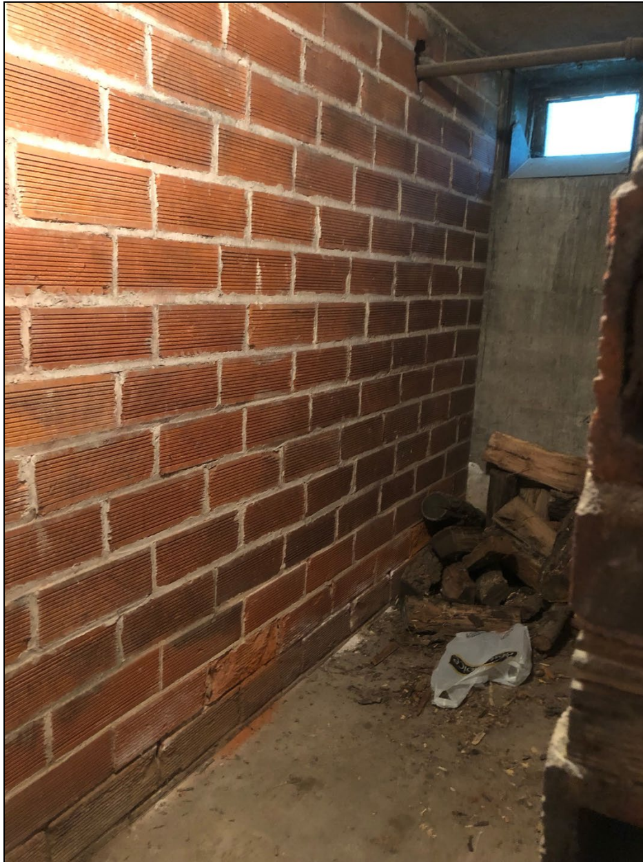
Figure 16: Basement level, wood storage room with chute to exterior; view facing southwest, 2022.
