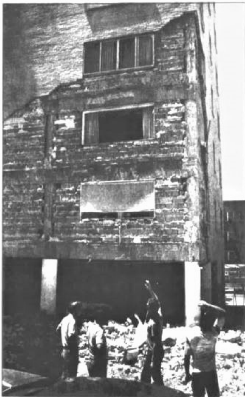
Figure 9. 1984 Image of Damage to the Northeast Corner of Sunset Tower. (Helliker, Kevin. "Brick Fall from Walls of Apartment Building; No Injuries reported." The Kansas City Times . May 14, 1984, 13. Newspapers.com.)
