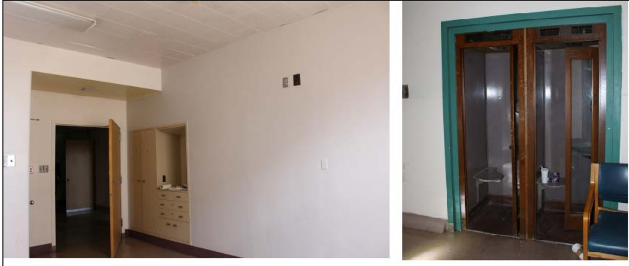
Figure 33: North Building patient room, left, and telephone booths. Federal guidelines did not go so far as to lay out specifications for phone booths... but they do mention that there should be phone booths ( Design and Construction of General Hospitals , 49), Photos by Elyse McBride, March 2017.
