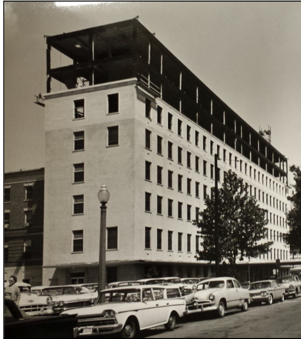
Figure 30: the differentiation of old and new brick above the fifth story is clear in this 1961 photo of the upper story addition to the Fowler Wing. Source: St. Luke's Hospital photo files.
