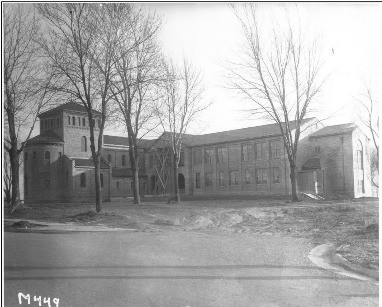
Figure 10. High School and Seminary under construction, 1930. Source: Missouri Valley Special Collections, Kansas City Public Library, Kansas City, Missouri.
