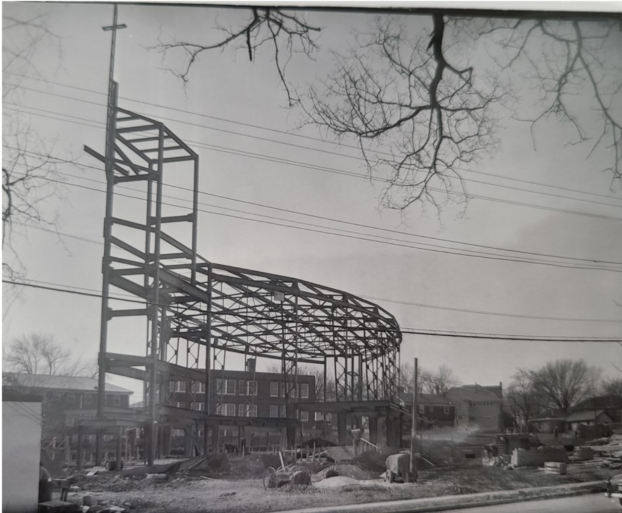
Figure 6. View looking south of the steel structural frame, February 1949. Source: St. Francis Xavier Parish Collection, Miscellaneous Photographs, Chancery Archives, Diocese of Kansas City-St. Joseph.
