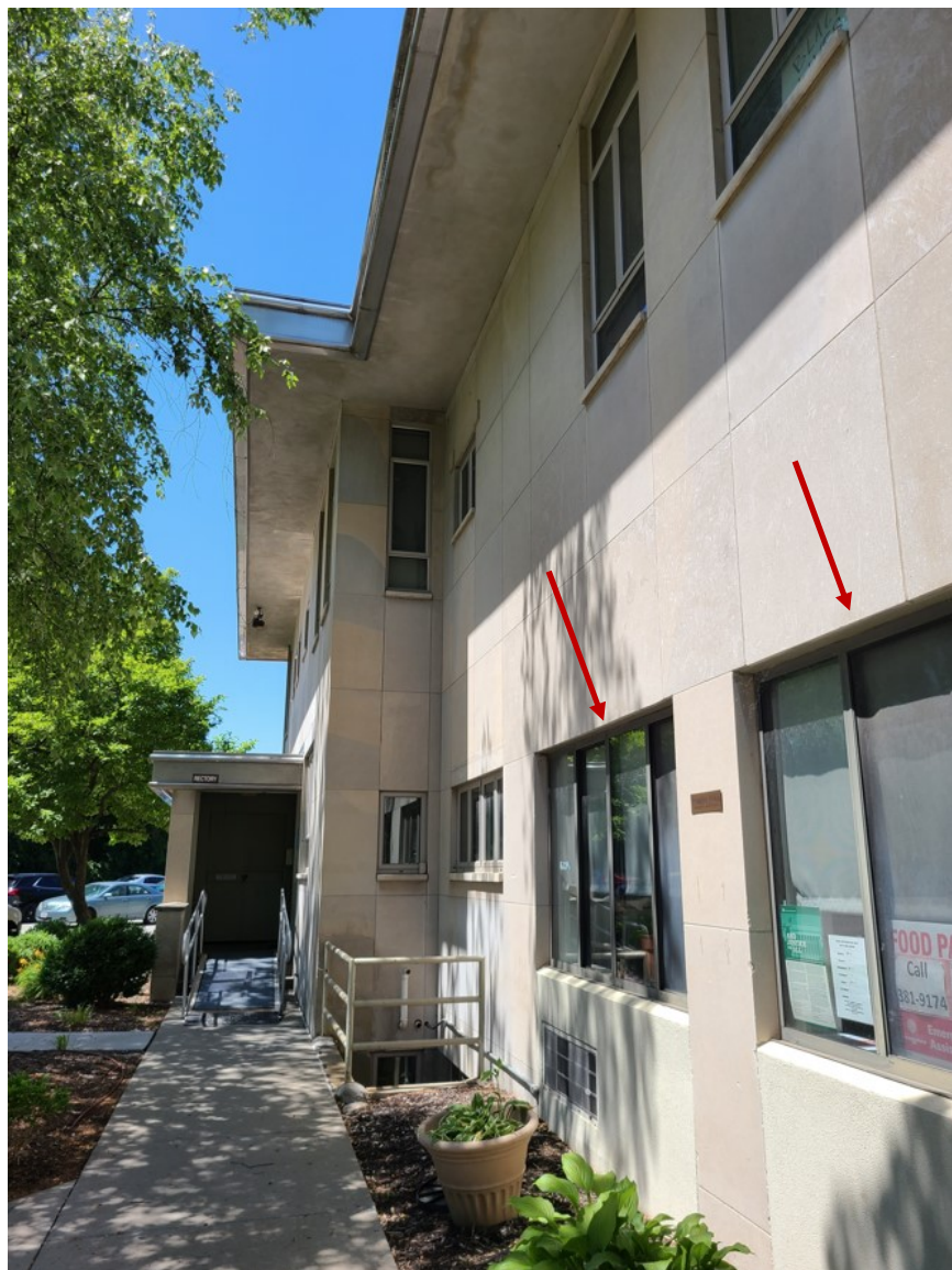
Figure 18. Partial view of the south elevation, showing the locations of the two former garage door bays (arrows). Source: Amanda Loughlin, June 2021.
