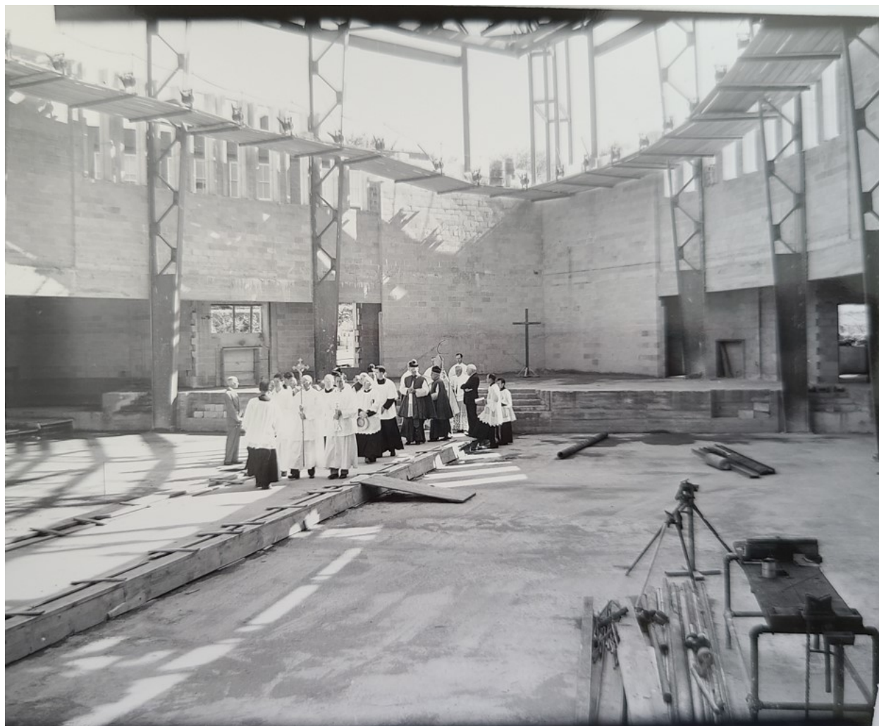
Figure 45. View of the Church wing under construction during the June 26, 1949 cornerstone ceremony. Source: St. Francis Xavier Parish Collection, Miscellaneous Photographs, Chancery Archives, Diocese of Kansas City-St. Joseph.
