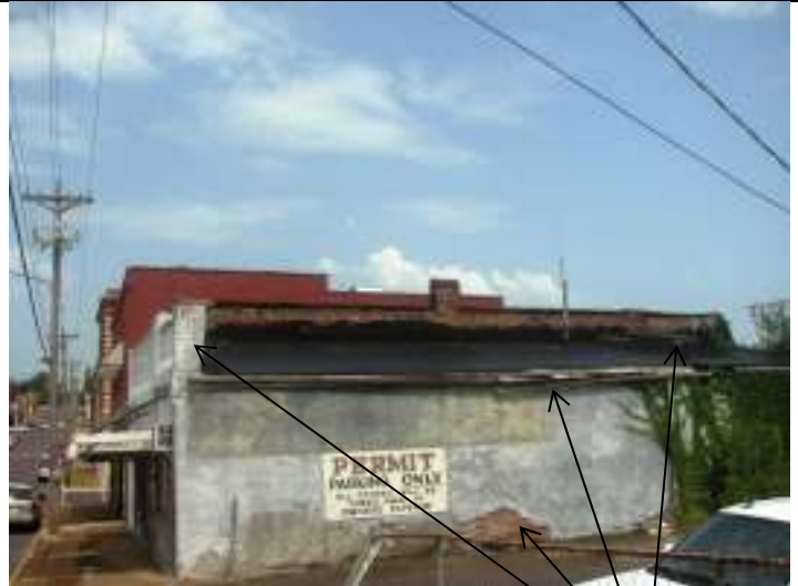
East elevation, showing missing stucco, leaning parapet, sagging roof, loose gutter, and cracks in brick roof ridge line
