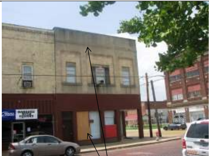
Façade (east), showing weathered stucco, and missing windows
