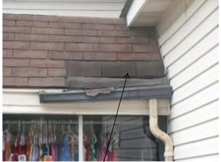
Façade; showing damaged roof
