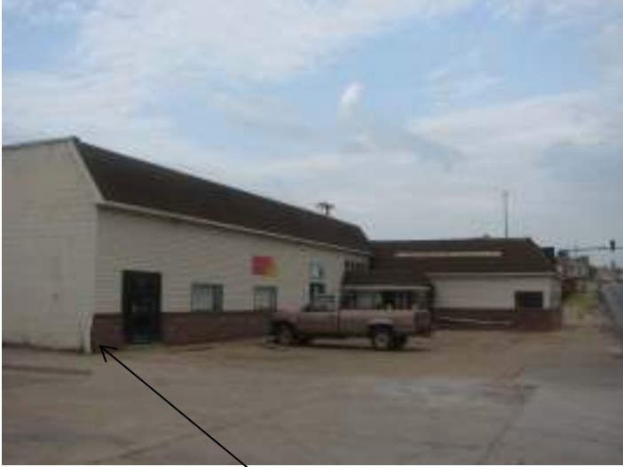
Façade and east elevation; showing damaged downspout
