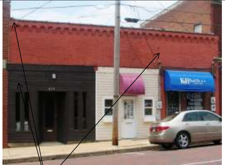
Façade, showing loose wood siding, loose (trim) coping, and areas of cracks in mortar
