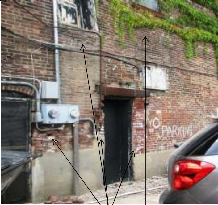
Rear (north) elevation, showing loose and fallen bricks, mortar issues, and vegetation on wall surface.
