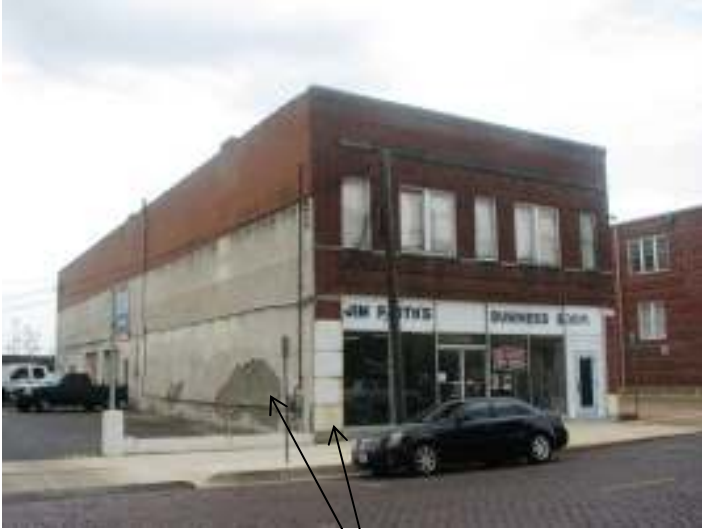
Façade (north) and east elevation, showing damaged concrete wall covering, weathered panels
