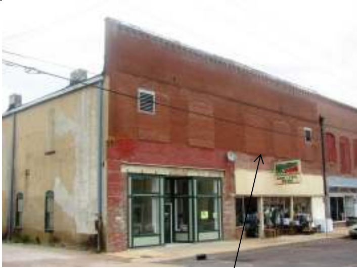
Façade (south) – 413 is second storefront from corner. Showing brick infilled windows
