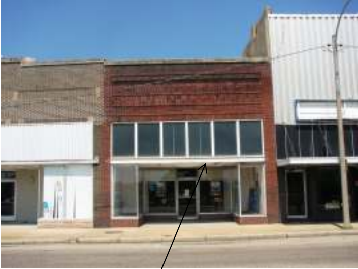
Façade (east), showing peeling paint
