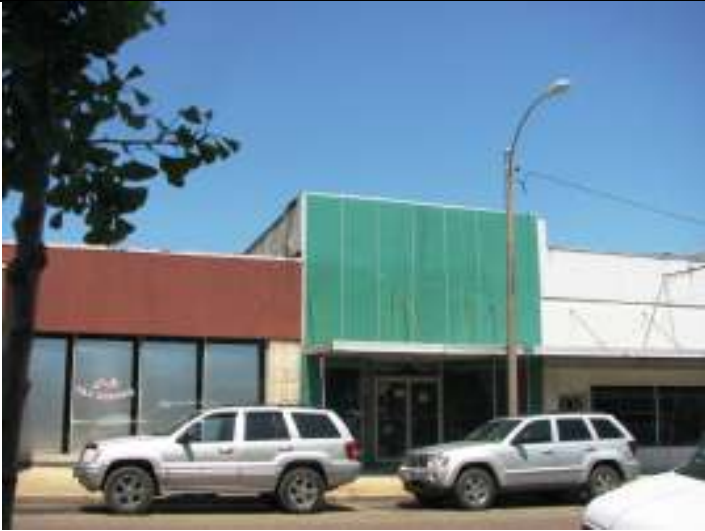
Façade (east) , some of the porcelain enamel panels are loose
