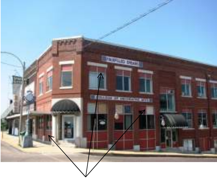
Façade (east) and north elevation, showing covered over windows
