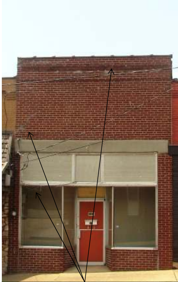
Façade, showing hanging wire, mortar repair of crack, and weathering of mortar
