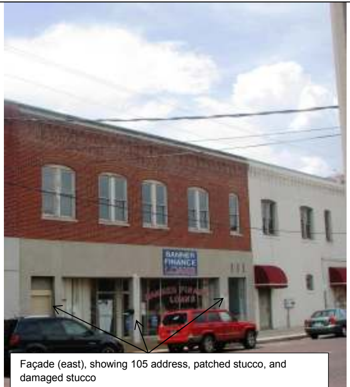
North elevation showing cracked stucco and missing stucco, with possible missing mortar
