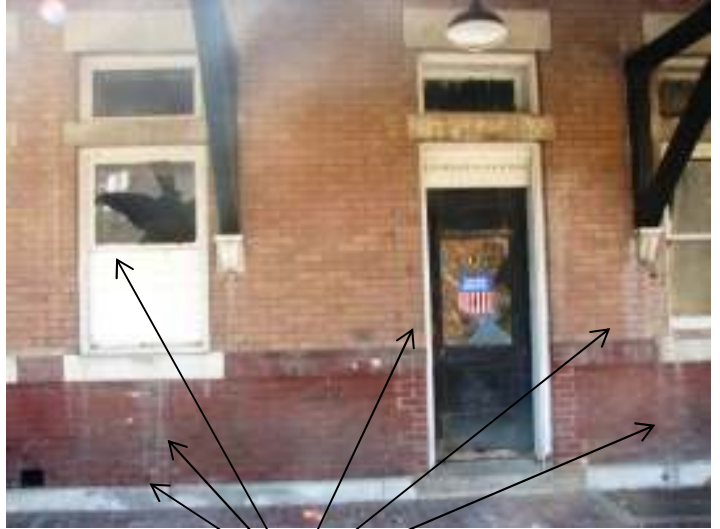
Façade (west), showing broken windows/glass, boarded up windows, missing mortar, and water damage to wall surface.
