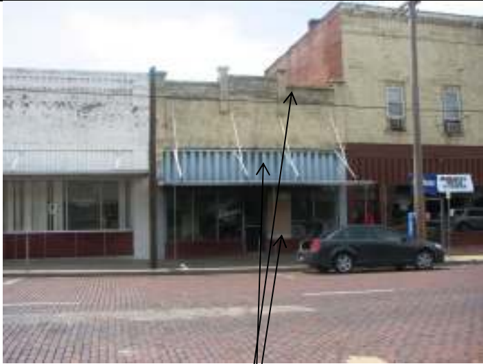
Façade (east), showing smoke damage on brick wall surface and awning, and missing store front window
