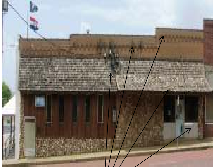
Façade, showing dent in bulkhead, loose/missing shingles, discolored bricks, wires/cables and cracks in brick wall surface.
