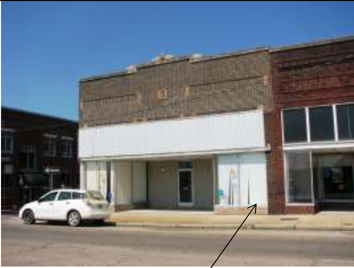
Façade (east), showing cracked window
