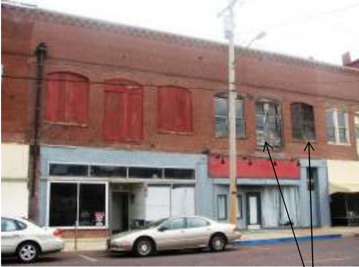
Façade (south) – showing boarded windows, deteriorated windows and doors
