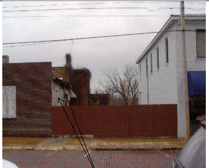
South elevation, deterioration of wood siding and roof rafters.
