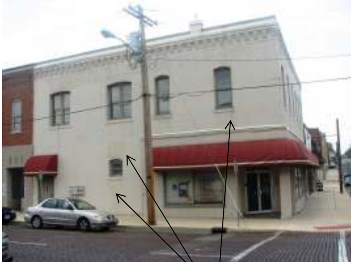
Façade (east), showing weathered stucco
