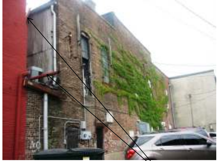
Rear (north) elevation – showing the west corner and disconnected downspout. Building is the red building in the photograph
