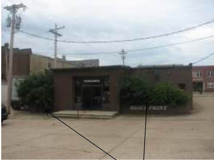
Façade (north), showing overgrown shrubs
