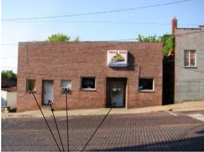
Façade (north), showing boarded up windows, and worn entrance doors.
