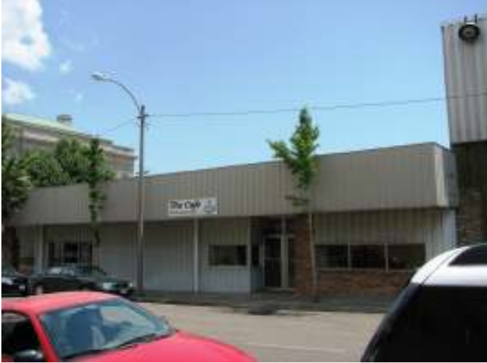
Façade (west) showing weathered metal siding
