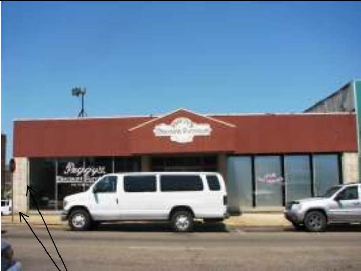
Façade, showing chip bricks, cracked foundation, and weathered sign.
