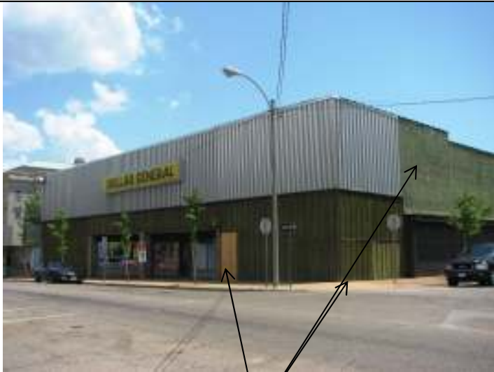
Façade (west) and south elevation, showing missing storefront window, deteriorated wood siding, and peeling paint
