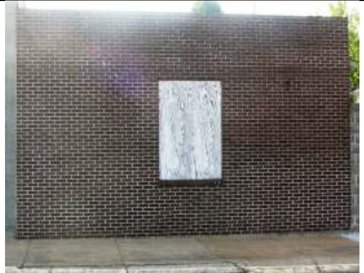
Façade – false front, showing boarded up window opening and no egress.
