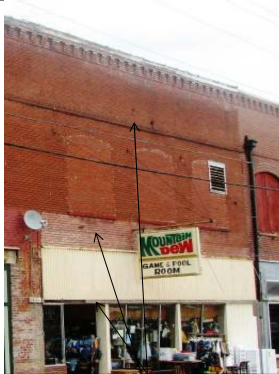
Façade – showing cracks in mortar, missing trim from metal slip cover and mortar issues
