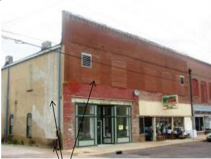
Façade (south) and west elevations – 415 is storefront on the left (end) – showing brick infilled windows, and deteriorated stucco. Water damage on lower section of west elevation
