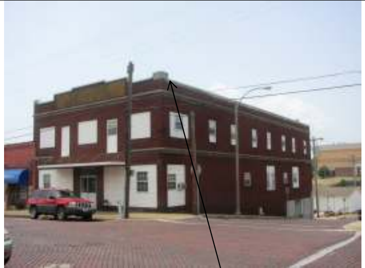
Façade and north elevation, showing improper re-pointing of brick and infill of windows
