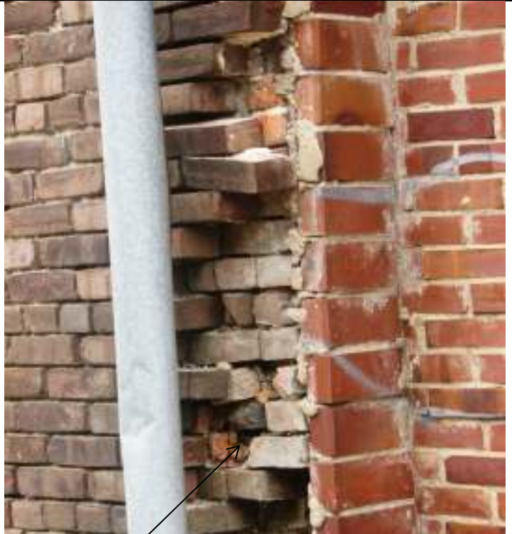
Loose and fallen brick on rear (north) elevation
