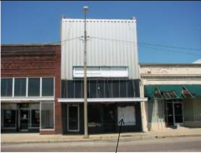
Façade (east), showing cracked storefront window
