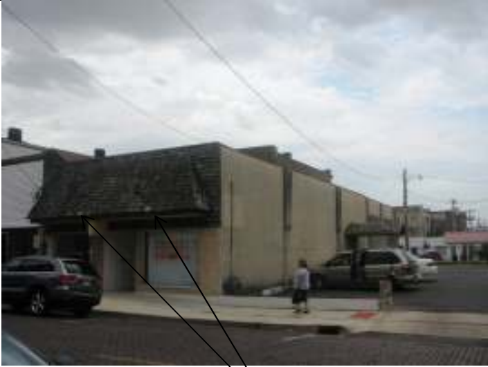
Facade (north), showing missing wood shingles
