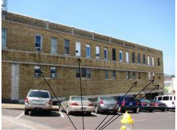
North elevation, showing boarded up windows, and missing windows, and vacant sign frame
