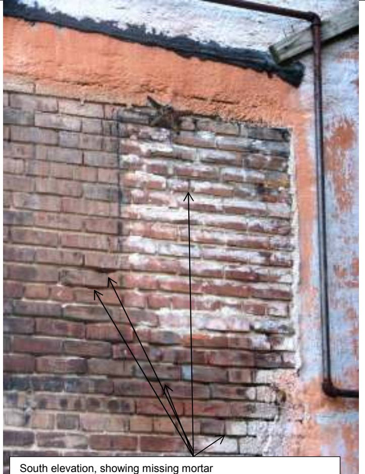
South elevation, showing missing mortar
