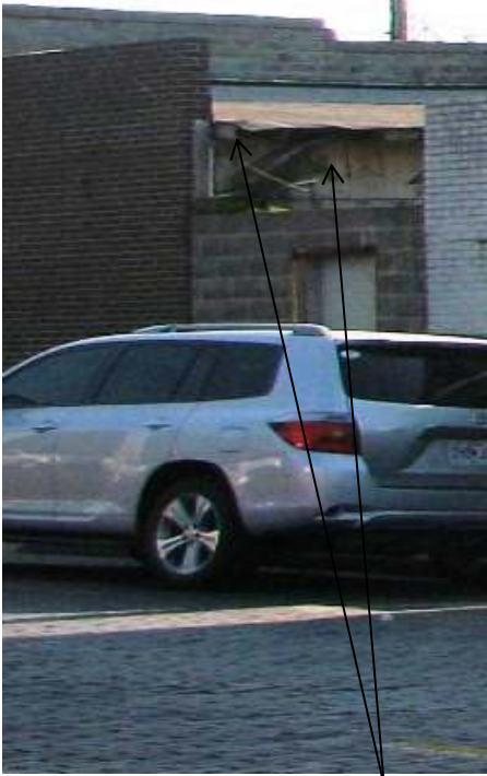
South elevation, showing the deterioration of the expose roof rafters and wall surface
