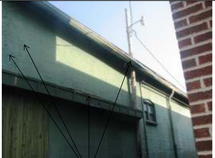
East elevation, showing bent gutter, deteriorated trim, and cracked brick wall surface
