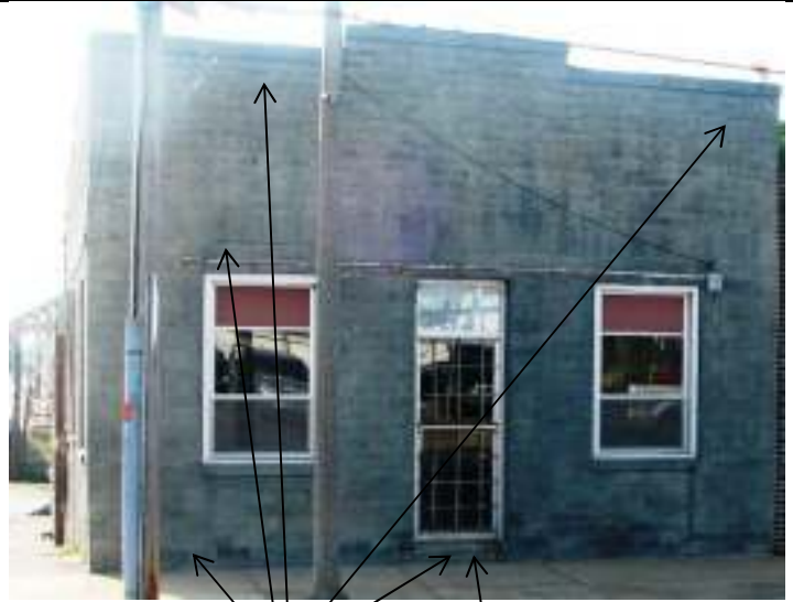
Façade, showing mortar issues, missing step and damaged screens.
