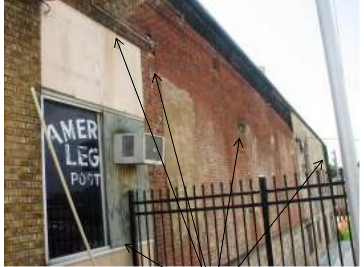
North elevation, showing crack in brick wall, boarded window, mortar issues, and vegetation on wall surface
