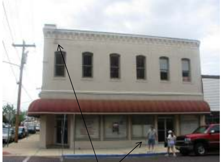
North elevation, showing weathered stucco
