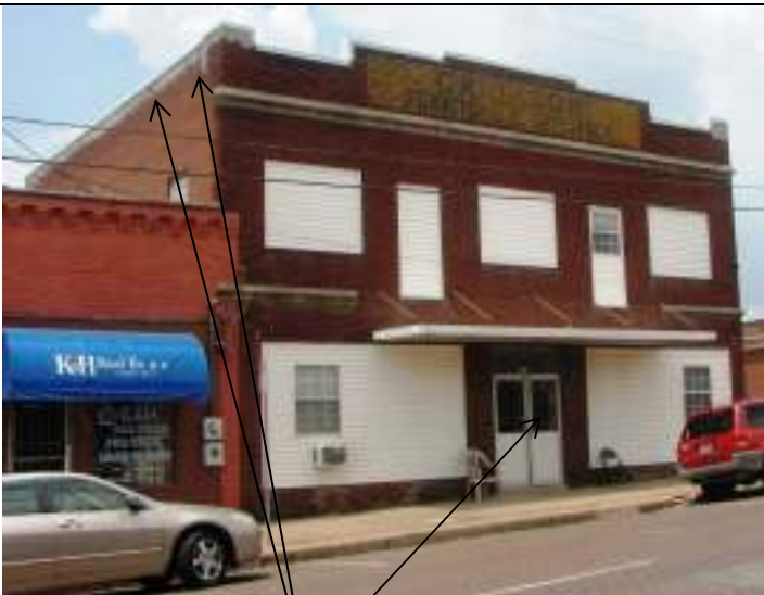
Façade and south elevation, showing improper re-pointing of the brick, missing brick, broken window in door, and enclosed window openings
