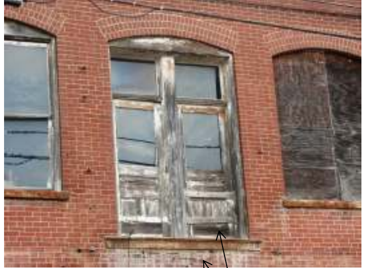
Upper level doors on façade and water damaged brick/mortar bellows doors
