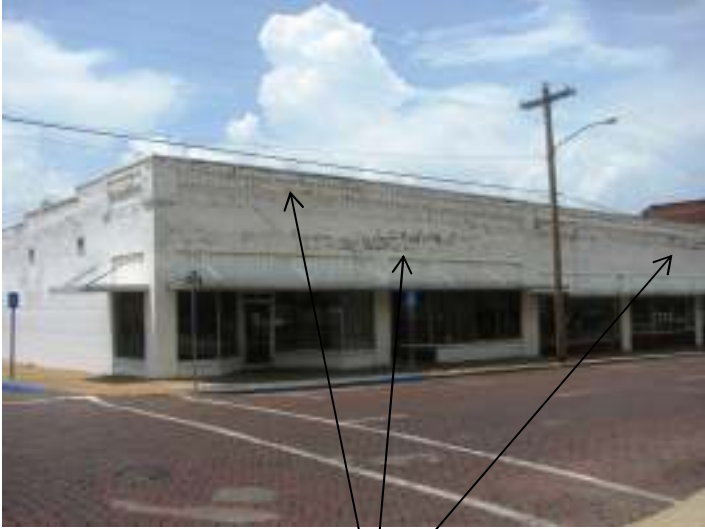
Façade (east) and south elevation, showing peeling paint and mortar issues
