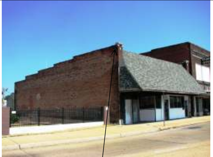
South elevation, showing loose brick
