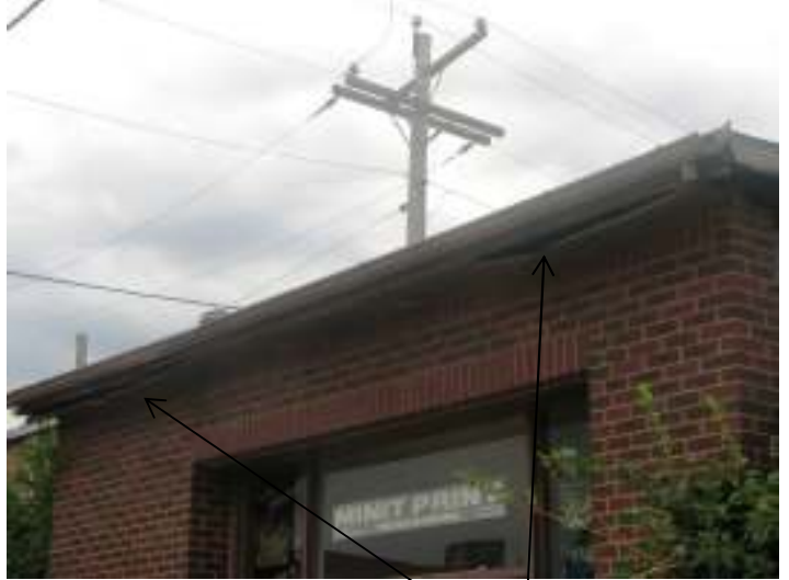
Façade, showing loose trim on the northeast and northwest corner of roofline
