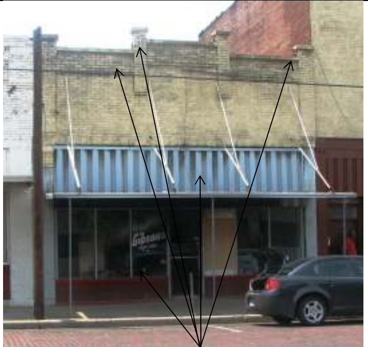
Façade, showing cracked window, missing mortar, and loose wires
