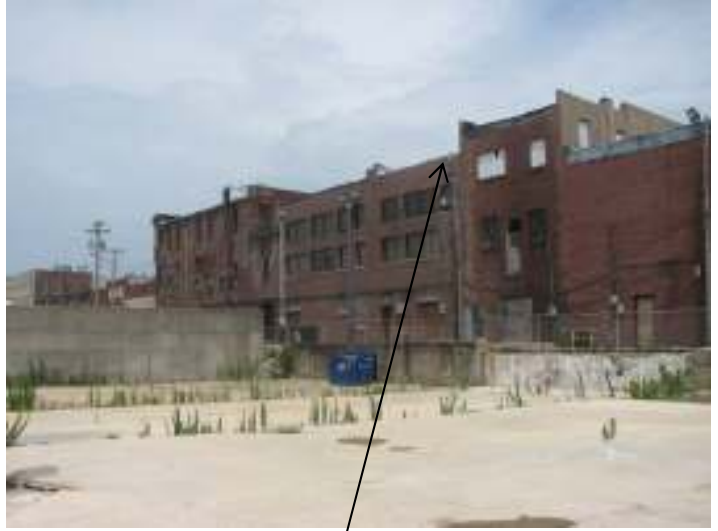
West elevation, showing previous brick work repair
