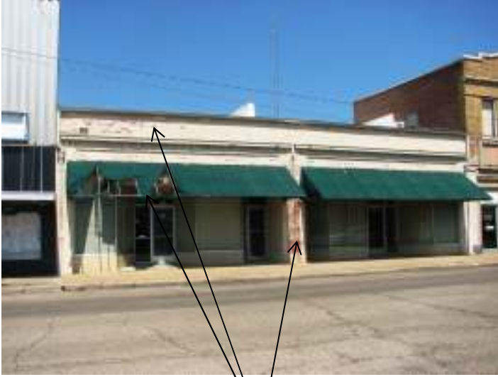
Façade (east), showing peeling paint, torn awning cover
