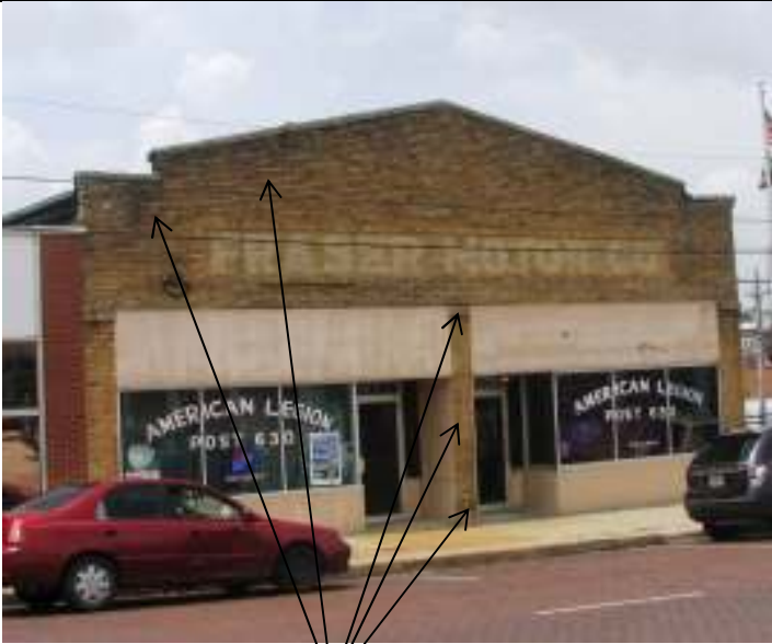
Façade, showing mortar issues
