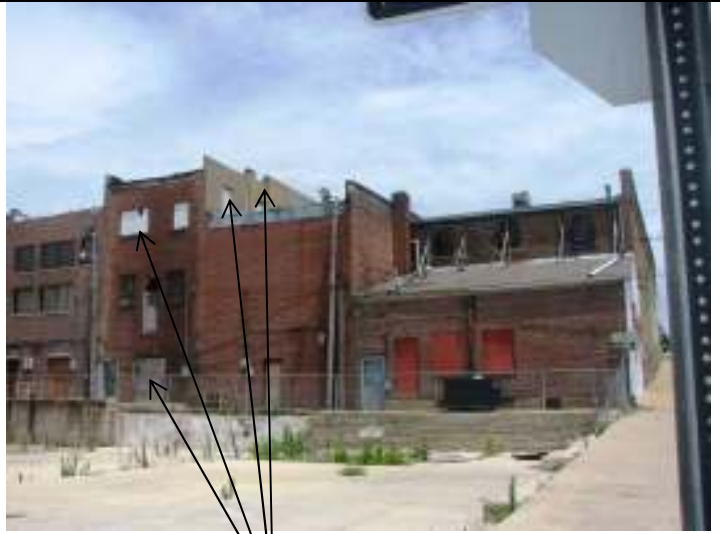
West and south elevations, showing boarded up windows and doors, and cracked stucco
