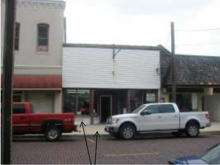
Façade (north), showing missing vinyl siding panel
