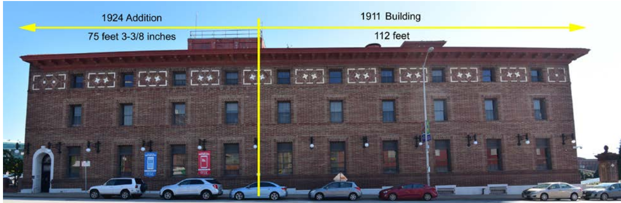
Figure 42. Annotated west elevation. Source: Brad Finch, f-stop Photography, annotated by Rosin Preservation.
