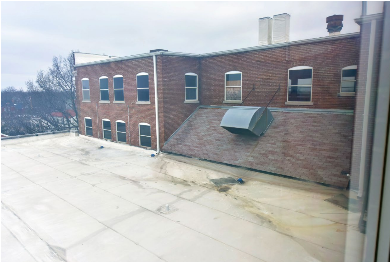
Figure 10. View from fourth floor, looking NW and showing the lightwell. Source: Brad Finch, January 2021.
