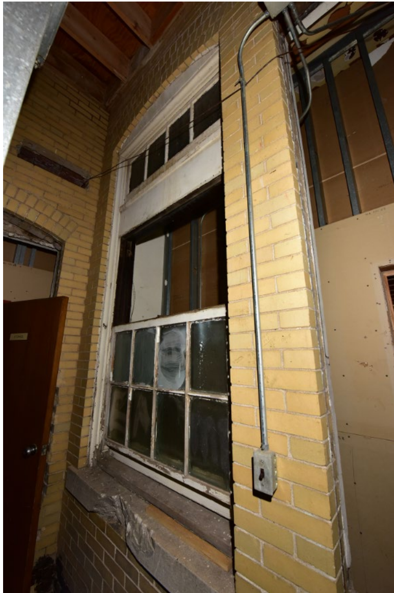
Figure 14. Lightwell to south of the former Boys' Lobby/current Meeting Room on first floor, looking NW. Source: Brad Finch, January 2021.
