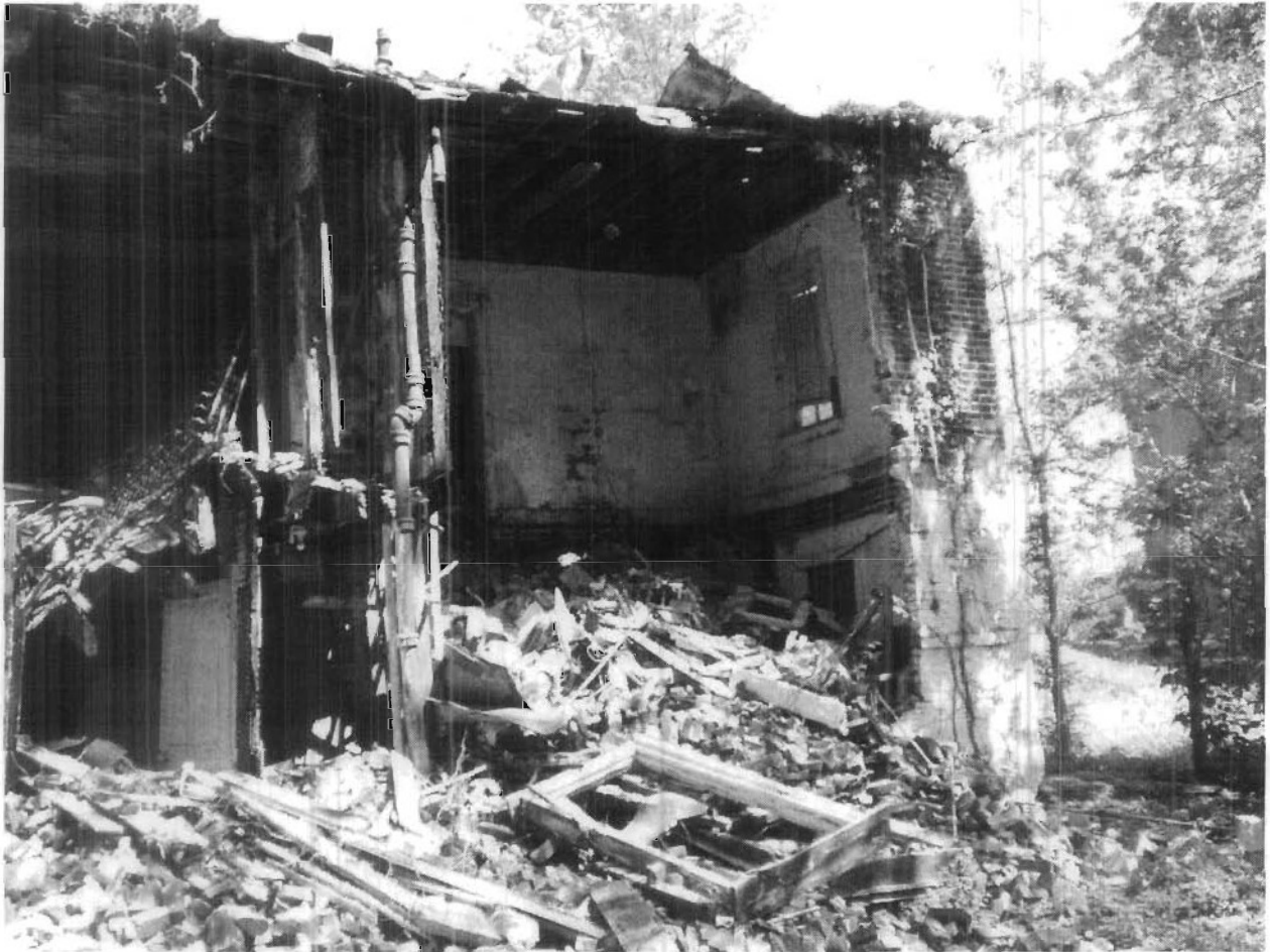
May 7, 2003; collapse of the rear addition
