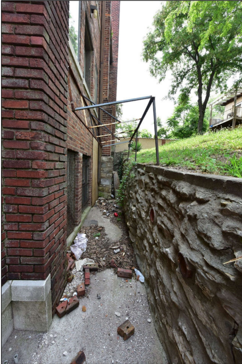
Figure 5. North side of the Hazelle, Inc. Building, looking west from Tracey Avenue through gate and showing the narrow gap between the building and the lawn to the north. Source: Brad Finch, June 2020.
