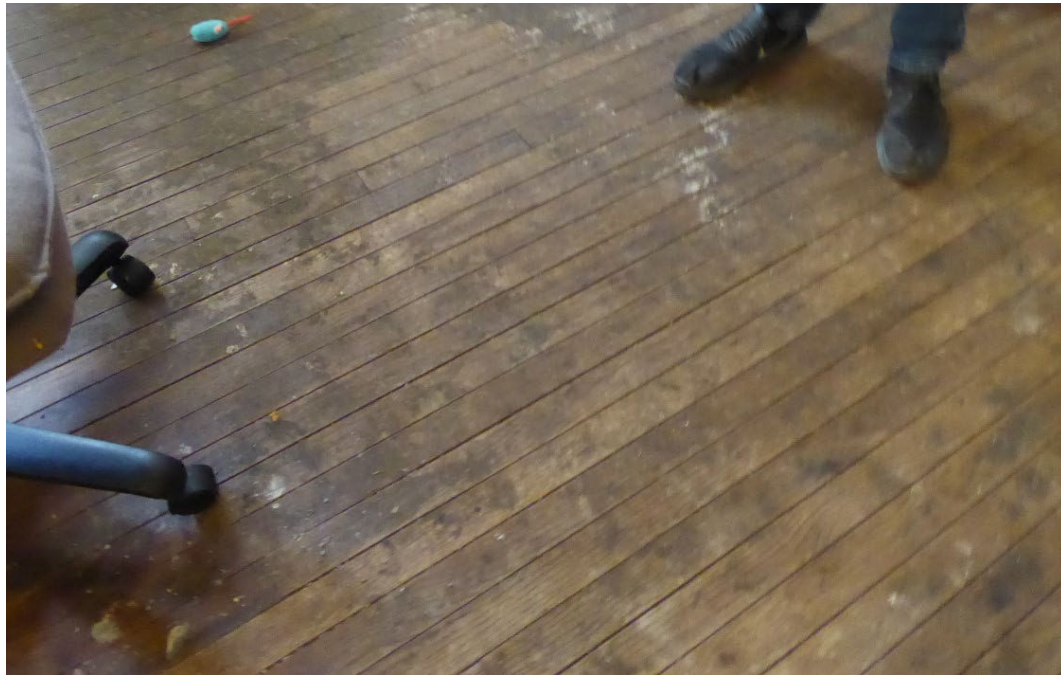
Figure 8. Example of historic wood flooring (top) and porcelain tub with non-historic flooring (bottom); photos taken in 5230 (top) & 5212 (bottom) East 12 th Street (Photos: Amanda Loughlin, April 2021).
