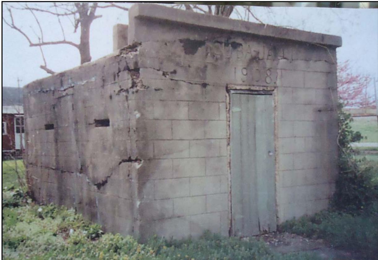
Figure 6: Historical Society photograph of building, circa 1970s. Note the condition and the exterior-most metal door (not original).
