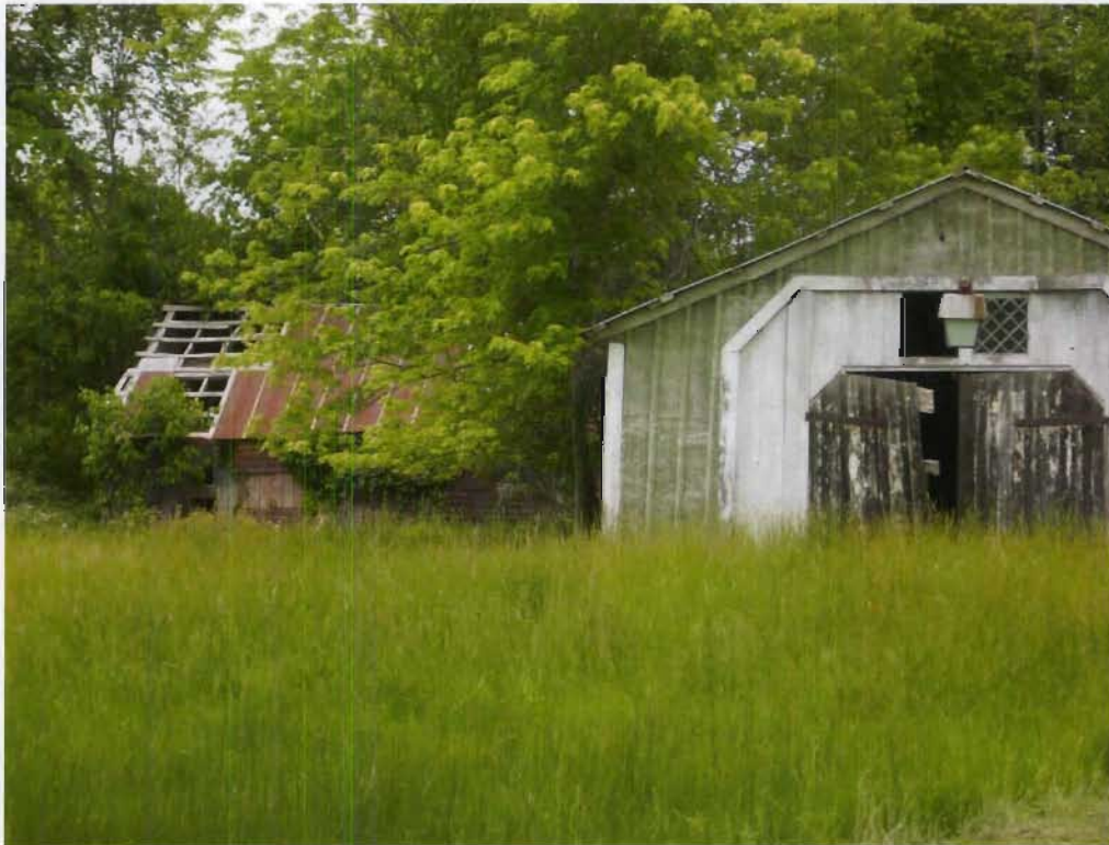
Structures 152c (Barn #2) and 152b (Green Barn #1), pictured from left to right, view N
