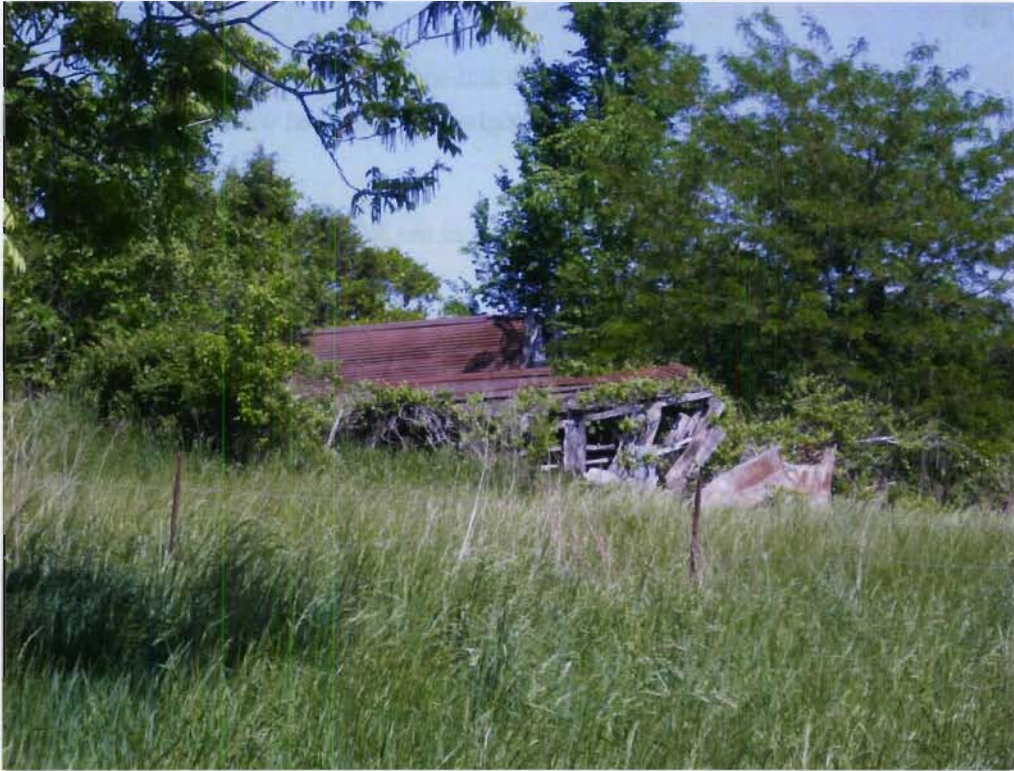
Structure 64d (Collapsed structure), view E
