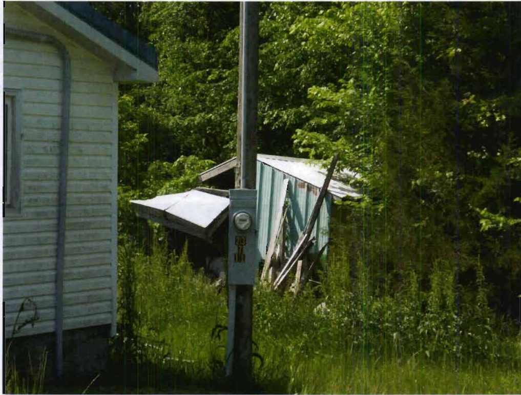
Structure 109b (Partially collapsed shed), view S
