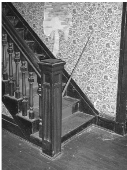
Staircase Details and Plaster and Lath Over Log Walls View to the Northeast
