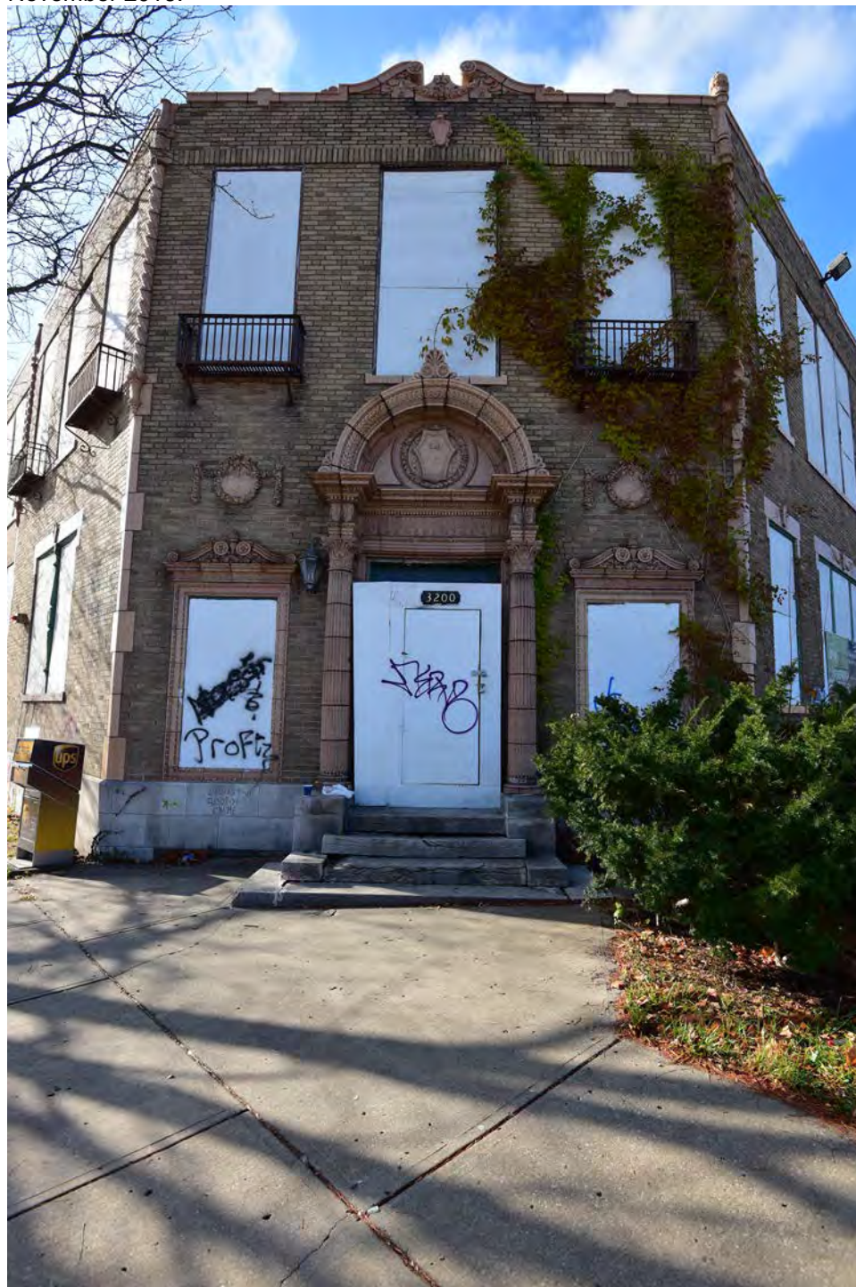
Figure 28. Entry of ACME Cleansing Company Building. Source: Brad Finch, F-Stop Photography November 2016.
