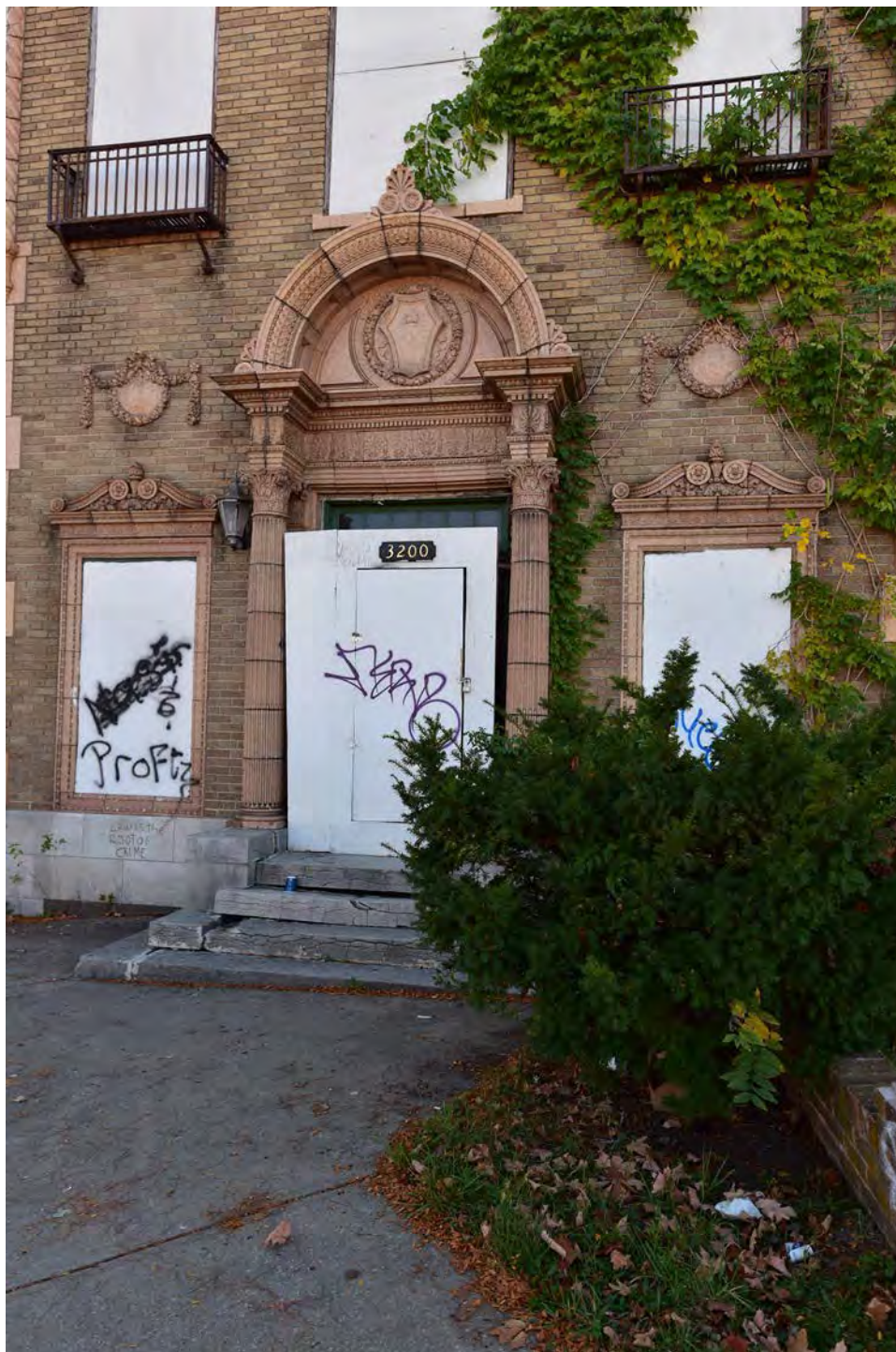
Figure 29. Entry detail of ACME Cleansing Company Building. Source: Brad Finch, F-Stop Photography November 2016.
