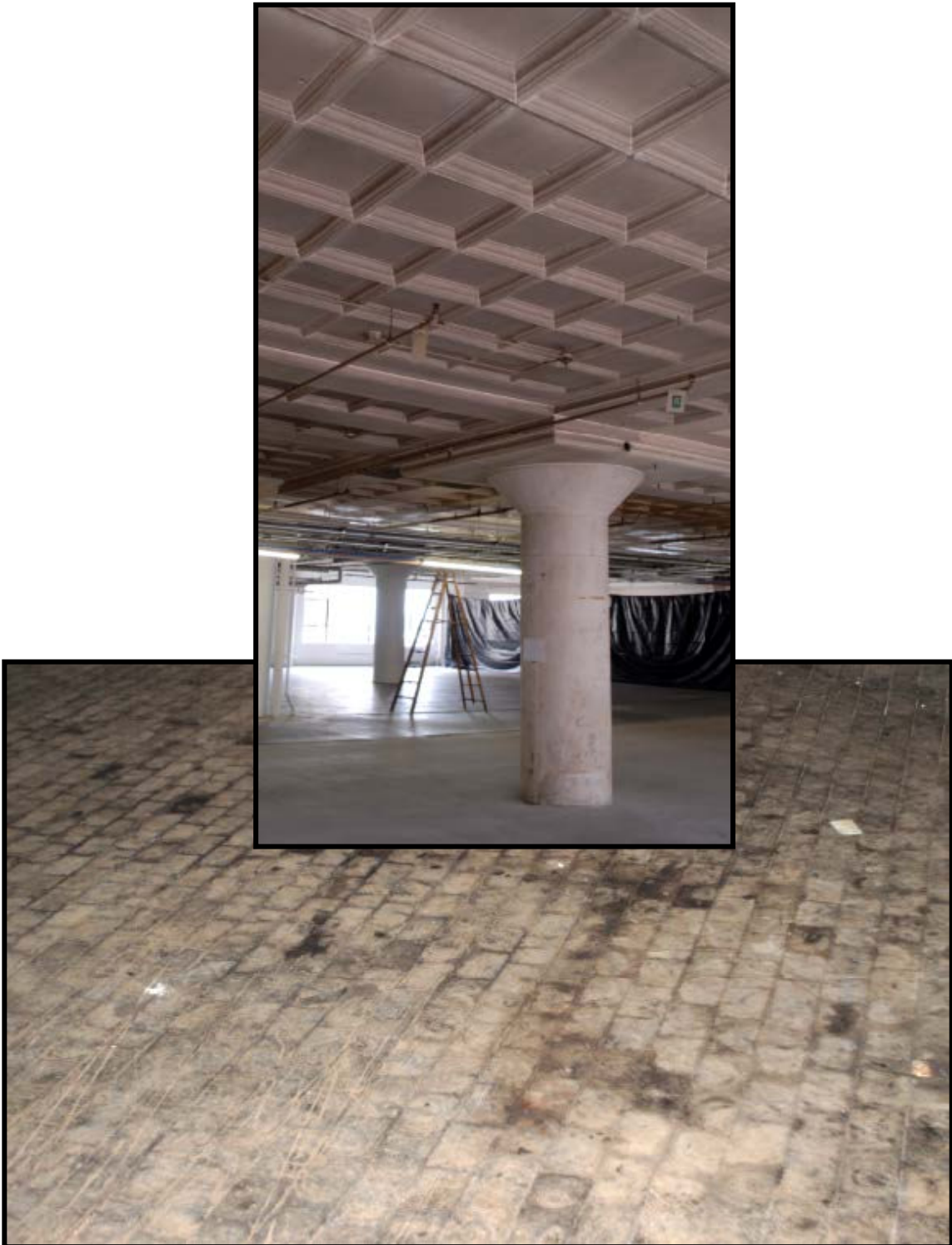
Figures 4A and B (top to bottom): Figure 4A illustrates the exposed concrete columns, floors, and monumental ceilings, Figure 4B is the first floor wood block flooring installed within the rear warehouse portions. Source: Matt Bivens, 2014-2016.
