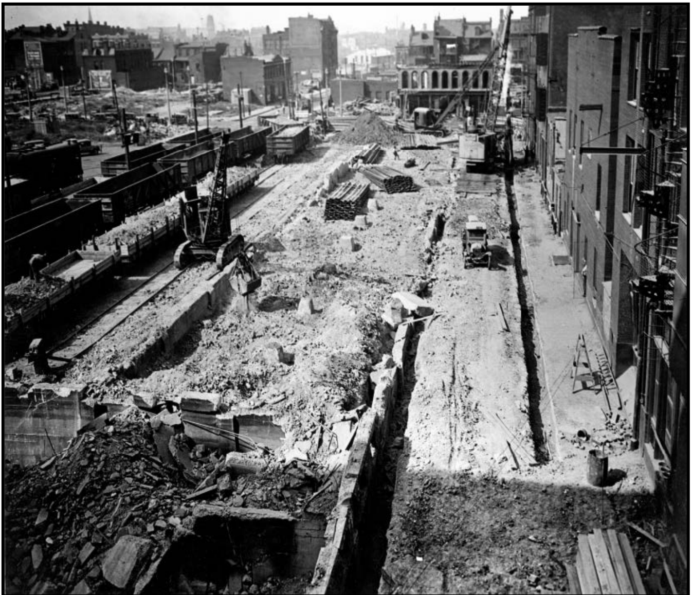
Figure 21: Photograph of site standing on Lucas Avenue between 12 th and 11 th Streets facing north, August 21, 1930. The exposed foundation is a portion of the former freight house. Source: Collection of Dale Jenkins, Illinois Traction Society.
