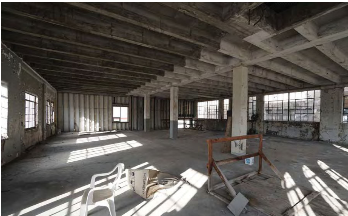
Figure 19: The second floor of the south unit, looking west, c. 1930 (above); and northwest, 2017 (below). Note the historic, character-defining features of the interior space vital to the significance of the property, are extant.
