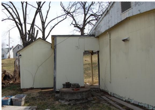
Figure 60: 217 Fair, c2018, covered well head
