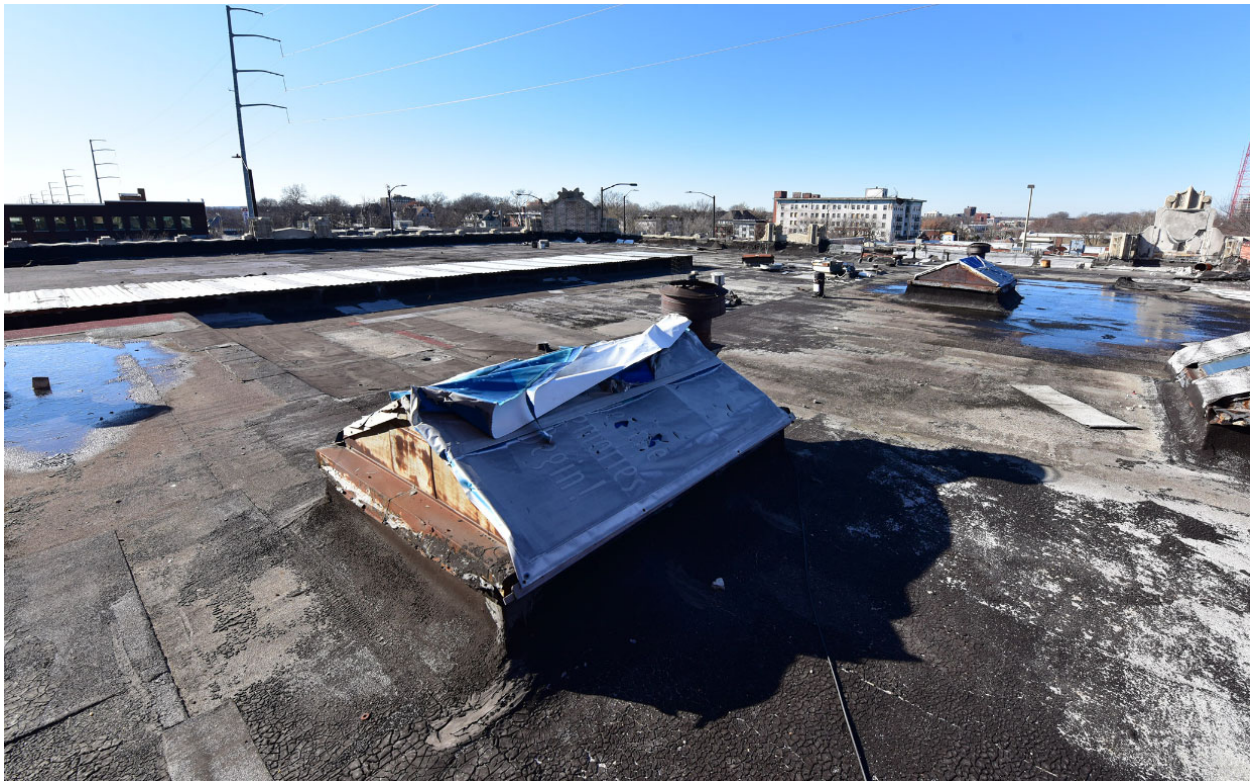
Figure 14. Roof and skylights over the two-story portion of the building, looking southwest from the northeast corner. Source: Brad Finch, December 2020.
