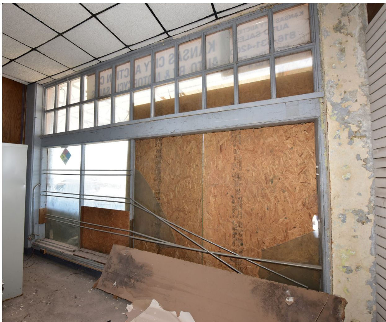
Figure 16. Extant historic storefront in west bay of historic south elevation. Source: Brad Finch, December 2020.
