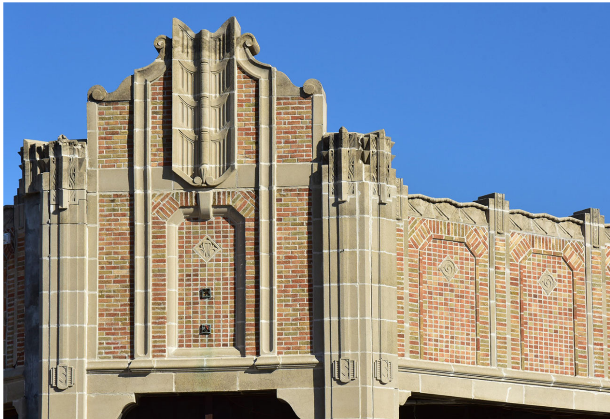
Figure 8. Parapet details on southwest corner and south elevation of canopy. Source: Brad Finch, December 2020.
