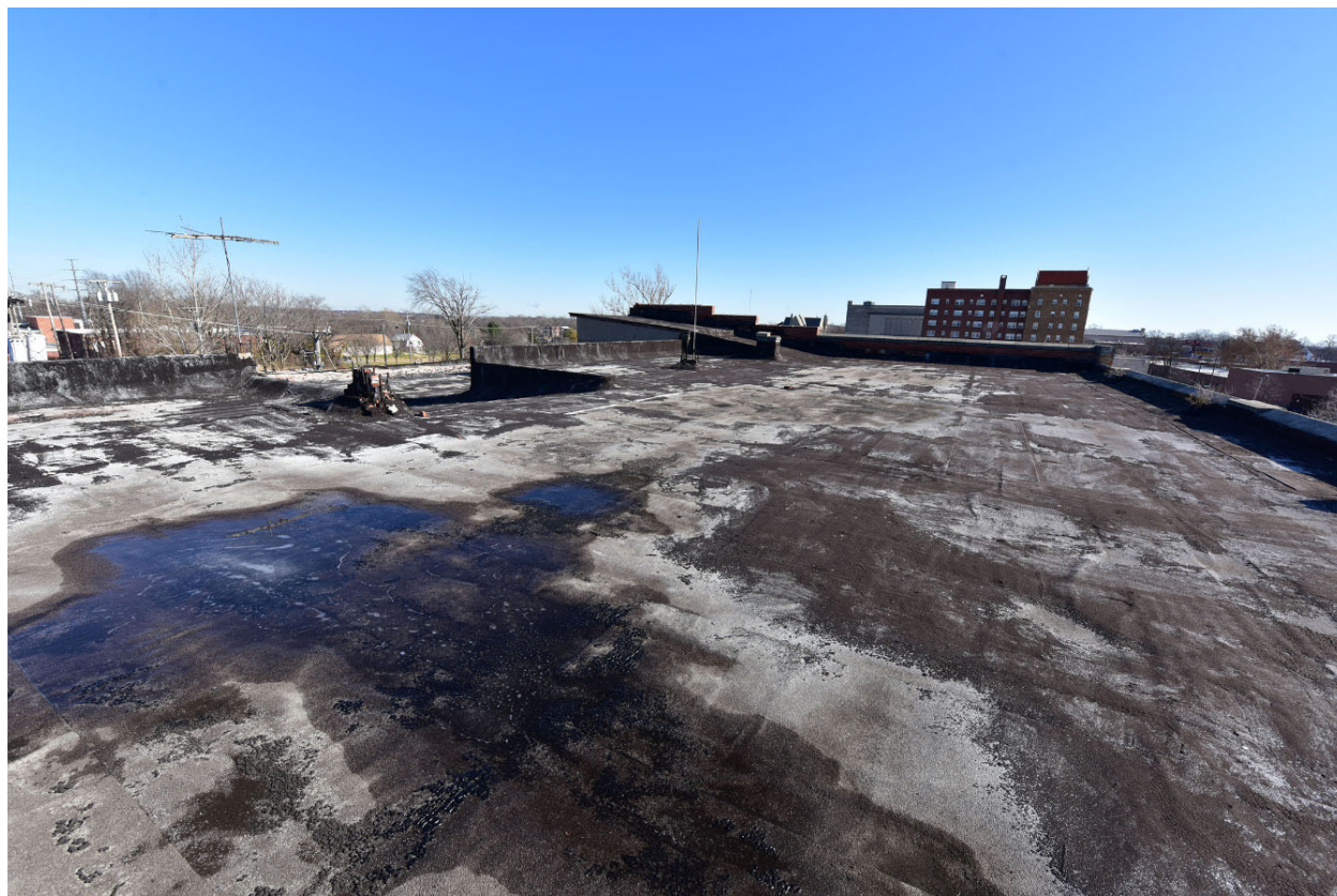
Figure 17. South (high) parking level of the parking garage, looking northeast toward ramp. The roof was historically exposed concrete but was covered with EPDM at an unknown date. Source: Brad Finch, December 2020.
