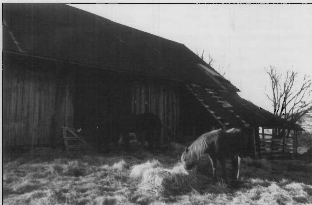
Cedarcroft's East Barn in 1993. The problems in the entry area are readily visible.
