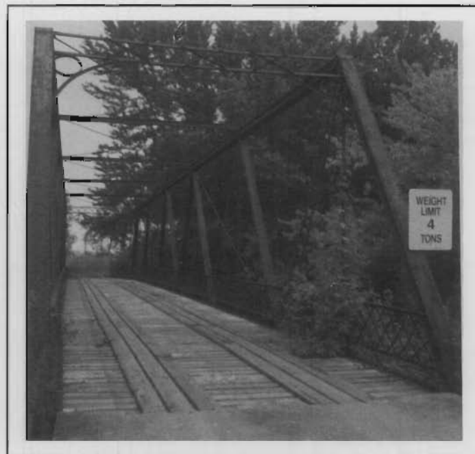
Henkins Ford Bridge, two miles north of Catawba, 1887, King Iron Bridge Company, Cleveland, Ohio.
