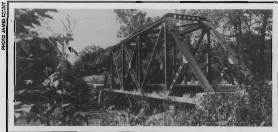
MKT Bridge #7 over the Little Bonne Femme Creek in Boone County is a Pratt through truss with riveted connections built by the A&P Roberts Company in 1898.
