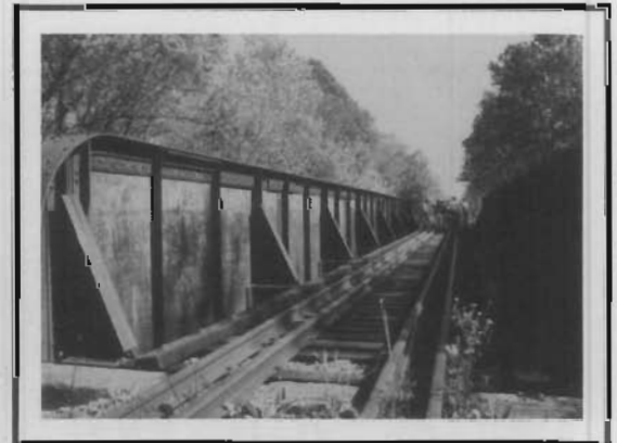
MKT Plate Girder (11) crossing the Middle Fork of the Tebo Creek in Henry County was built as a through girder by the Wisconsin Bridge and Iron Company in 1925.
