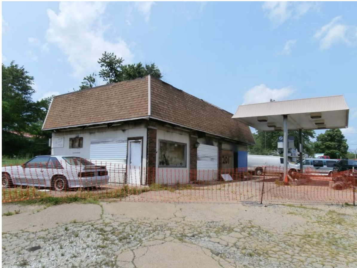
Figure 18. 201 S Front Street within the former city boundaries of Elvins appears out of use and recently suffered fire damage. Photographed by Amber Cox, June 1, 2019.
