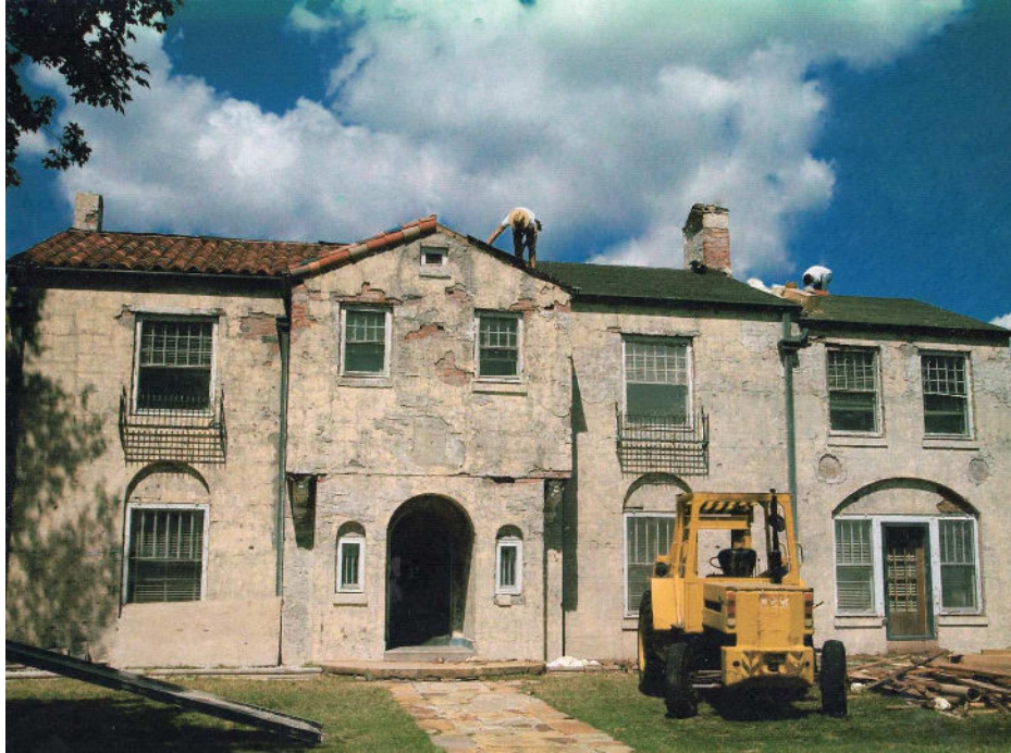
Figure 30: South elevation facing north during the 2006 exterior renovations. The original clay roof tiles were removed, restored, and reapplied. The exterior stucco was replaced. The windows and gutters were removed, and replaced with replicas that matched the original 1926 elements. Courtesy of MSSU Archives
