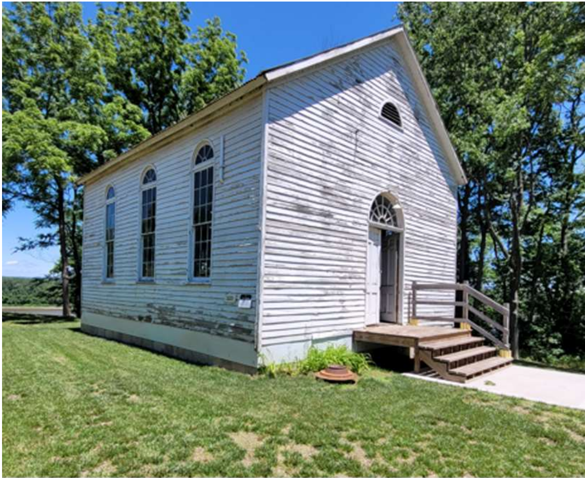
Above: The Anna Bell Chapel today with its new foundation and a new front porch; the privy has also been lost. Most of the remaining materials are original, including the lap siding and arched windows seen here, as well as interior features.
