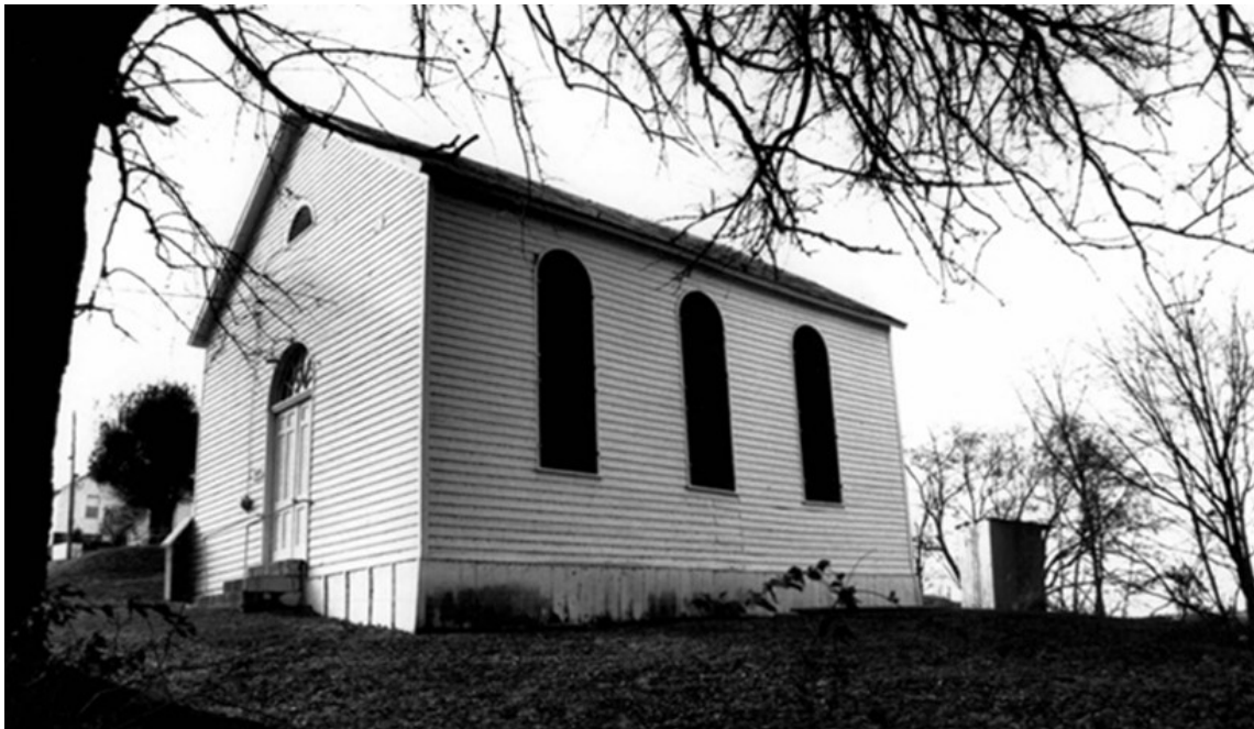
Above: The Anna Bell Chapel ca. 1992 when it was listed in the National Register. The privy (at right) was still standing, and was listed as a contributing resource.
