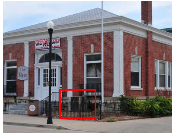
Example of a mechanical unit inappropriately located on the primary façade, 339 East Broadway, 2014.
