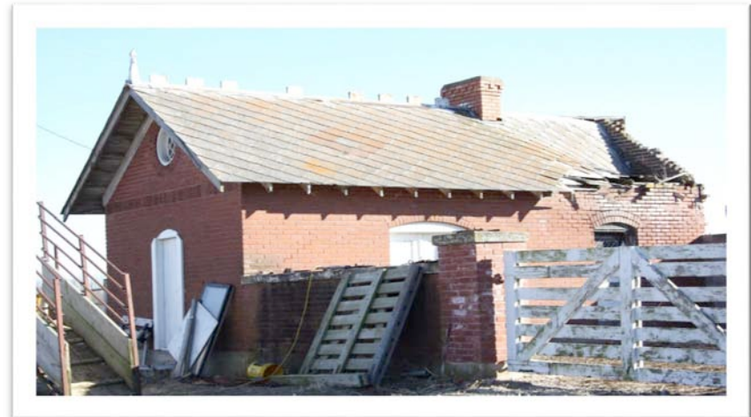
Top: View of mothballed house, ready for rehabilitation. Lawrence, KS, 2009. Below: View of structurally unsound roof structure on a historic outbuilding. The rest of the structure is in good condition, therefore only select demolition of the deteriorated roof structure is needed and can be repaired and saved. Boonville, MO 2009.
