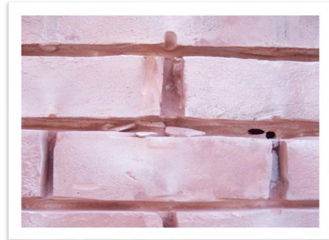
Incorrect mortar removal has caused permanent and irreparable damage to the historic brick, Kansas City, Missouri, 2009.
