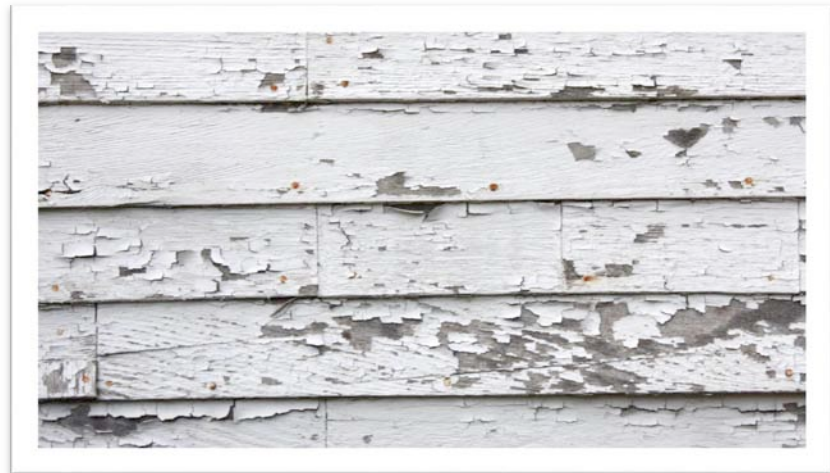
Example of cracked and peeling paint in need of repair. Loose paint should be carefully removed prior to priming and painting, Harrisburg, Missouri, 2008.
