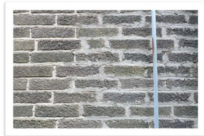
Incompatible Mortar Joints. New mortar installation (right side of the picture) does not match the original (left). Repointing has left mortar on the face of the brick.
